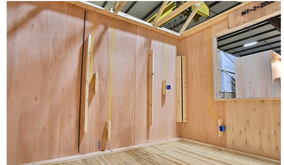
Quick dry-in of the structure's envelope and open cavity design simplifies MEP installations
